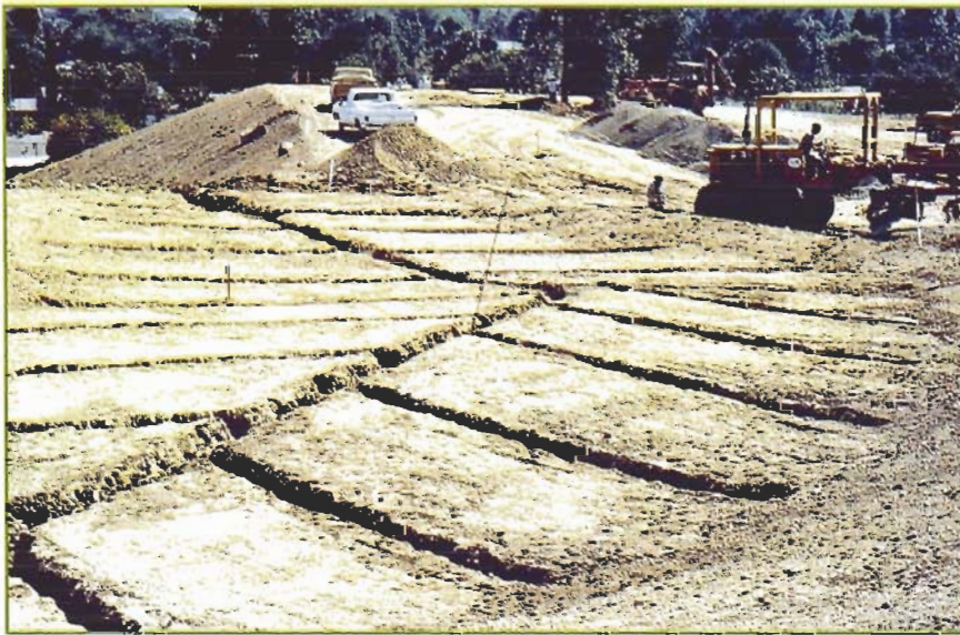
Figure 2 – Lateral lines should be spaced not more than 15 feet (5m) apart and have a natural fall to the mainline of at least 0.5%.
